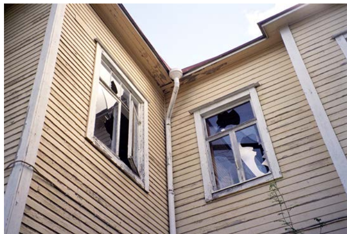
Broken windows expose the homes interior to outside temperatures.
