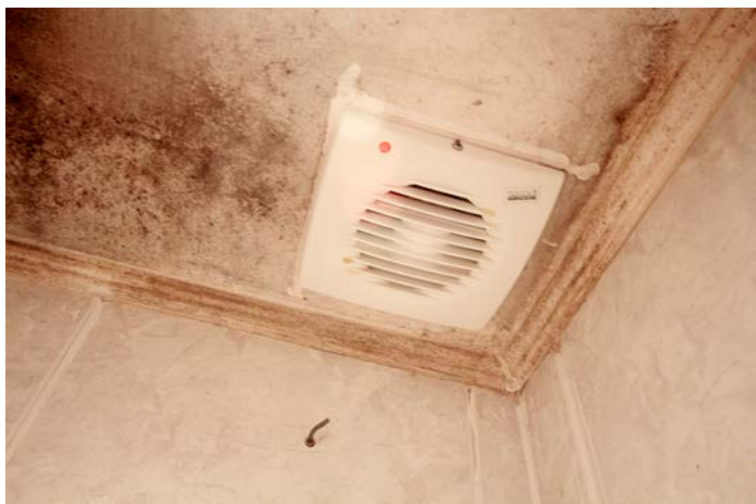
Mold is evidence of an improperly vented exhaust fan.
